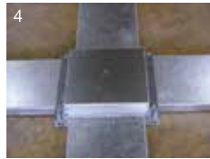
4 Fasten the trap frame, side blanks & ensure all the ductings and junction boxes are secured
